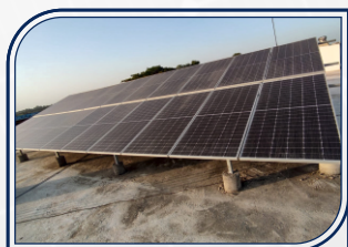
25 KW Vijapura Motors — Himmatnagar, Gujarat —
