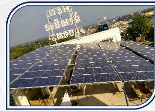
40 KW Hotel Paramount — Tarapur, Gujarat —
