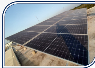
15 KW Metro Diesel — Himmatnagar, Gujarat —
