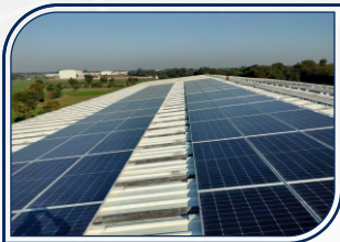
100 KW Ambika Cold Storage — Vijapur, Gujarat —
